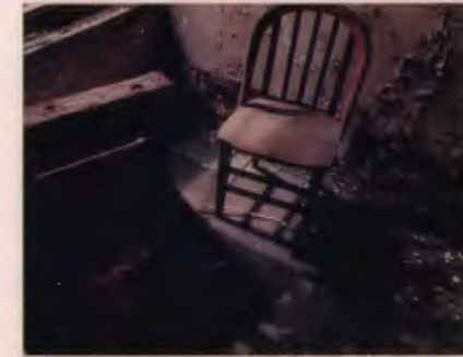
The Great Hall on Ellis Island is a hollow ruin; passageways are overgrown with vegetation, rooms vandalized, walls crumbling in decay.
