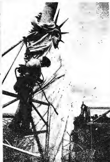
The last of the 500-member work crew employed on the renovation takes down the world's tallest scaffolding.
