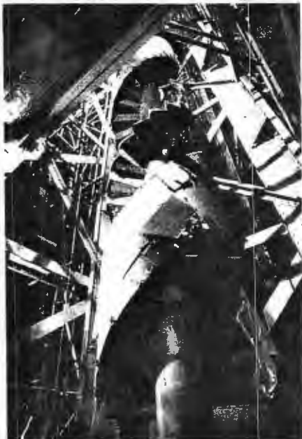
A new spiral staircase with rest areas and observation platforms leads to the diadem.
